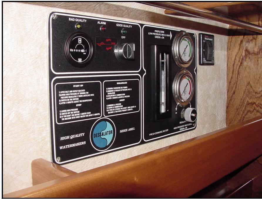
Picture 11 – Desalinator control panel
