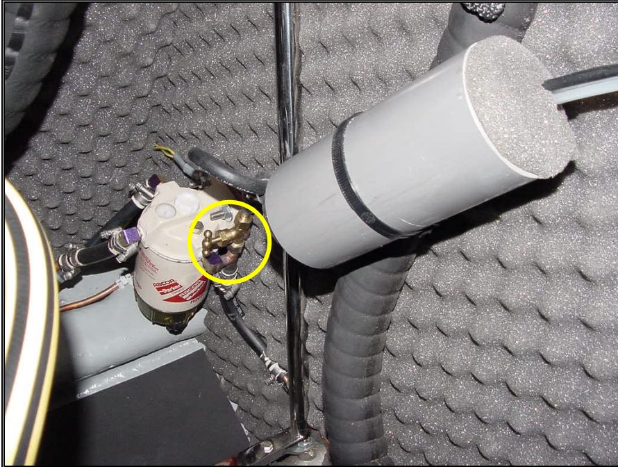
Picture 18 – Shutoff on the decant filter
