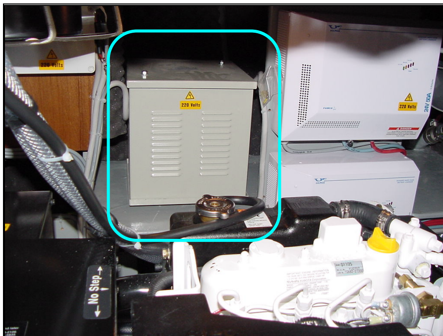
Picture 39 – 110 / 220 V transformer
