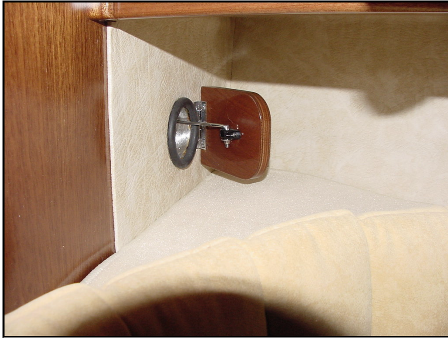
Picture 16 – Warmed air outlet in the fore cabin
